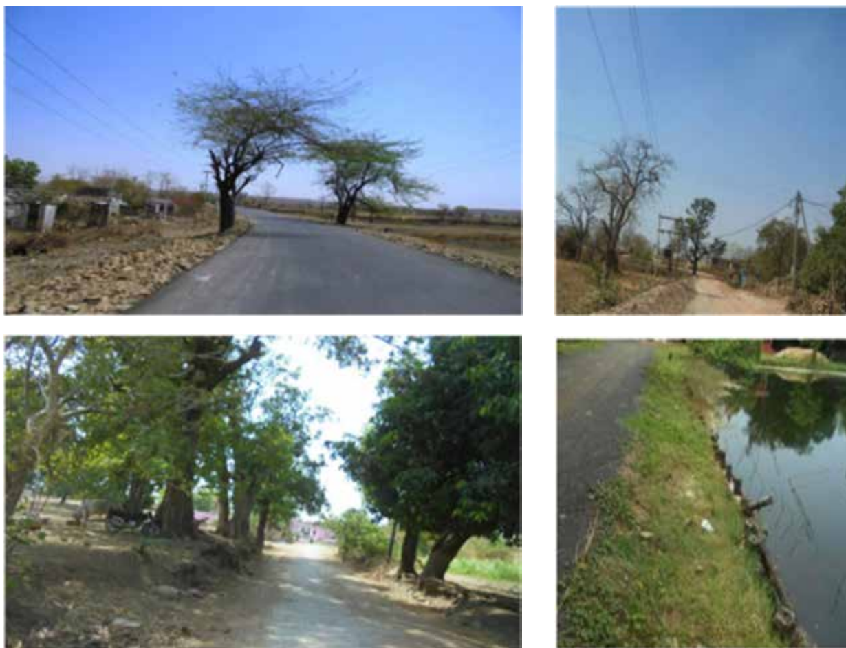
Figure 3-6: Insufficient or Poorly Maintained Shoulders
