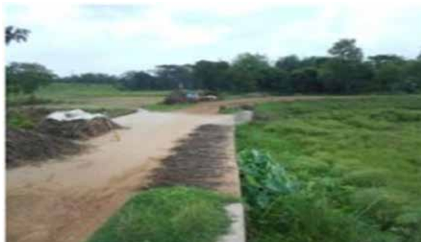
Figure 3-4: Unsafe Cross Drainage Structures
