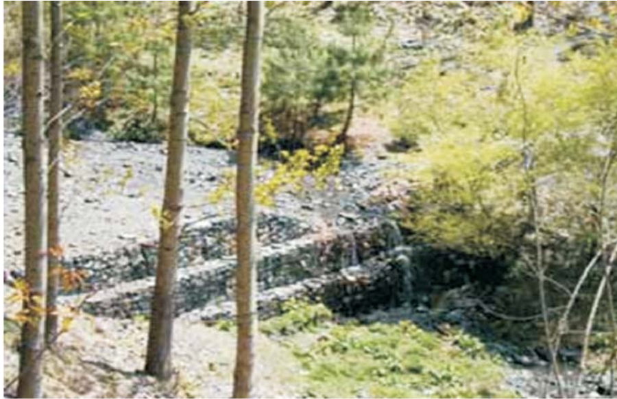
Three tiered gabion check dam
