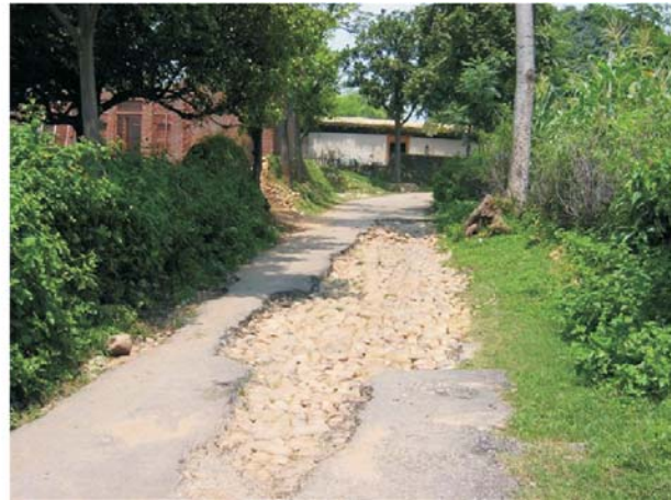
Section of same road without proper side drains
