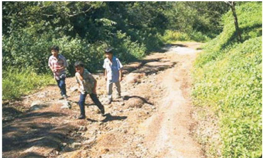
Adverse environmental impact from road surface erosion caused by steep road grades and insufficient cross-drains. This road is also difficult to maintain
